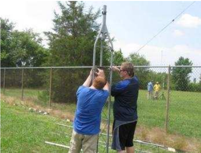
Nathan Hatchel, KK4FRP , and Josh Steele, KB3VHK , getting the tower ready while Ted Bertrand, KI4WPX and Thomas Styron, KB7L , set up the Tarheel Screwdriver in the background.
