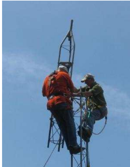
Murray, K4MHM, and Terry, K4ZYD, remove top section of tower and lower it to the ground. Photo by W4YDY
