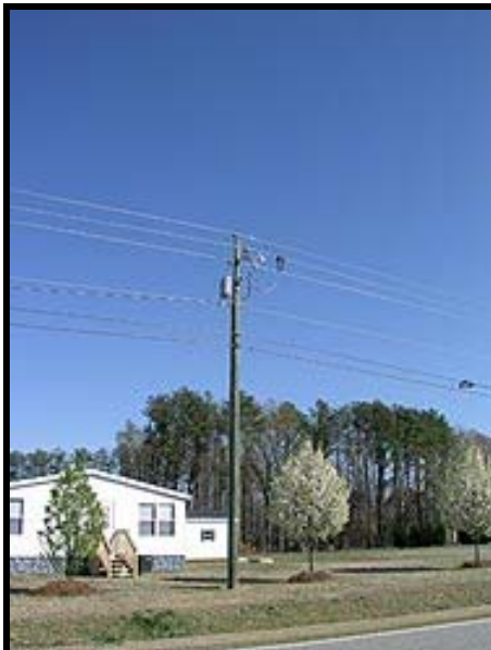
A pole-mounted BPL extractor in the Progress Energy Corp system. [Gary Pearce, KN4AQ, Photo]
